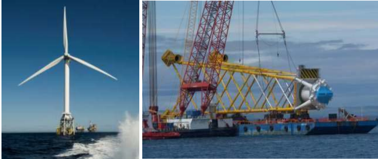
Figure 5-7. Repower 5-MW turbine installed on jacket substructure (left, Talisman Energy, NREL/PIX 17883) and load-out to Beatrice Field (right, Talisman Energy, NREL/PIX 17884)
